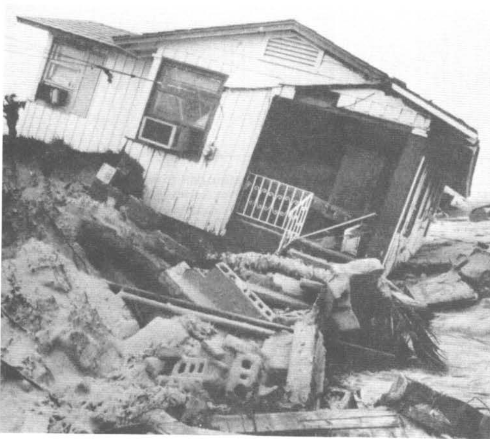
Flood water velocity produces lateral forces that can cause scour and result in collapse of foundations (above left), increase the magnitude of debris impact loads (below left), and dislocate buildings from their foundations (below).
