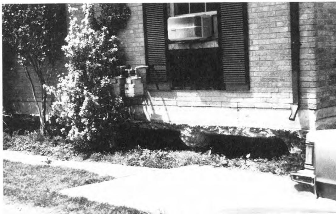
Figure 9-3. Subsidence on organic soils has resulted in structural damage to this house in New Orleans. Source: B. Cox.
