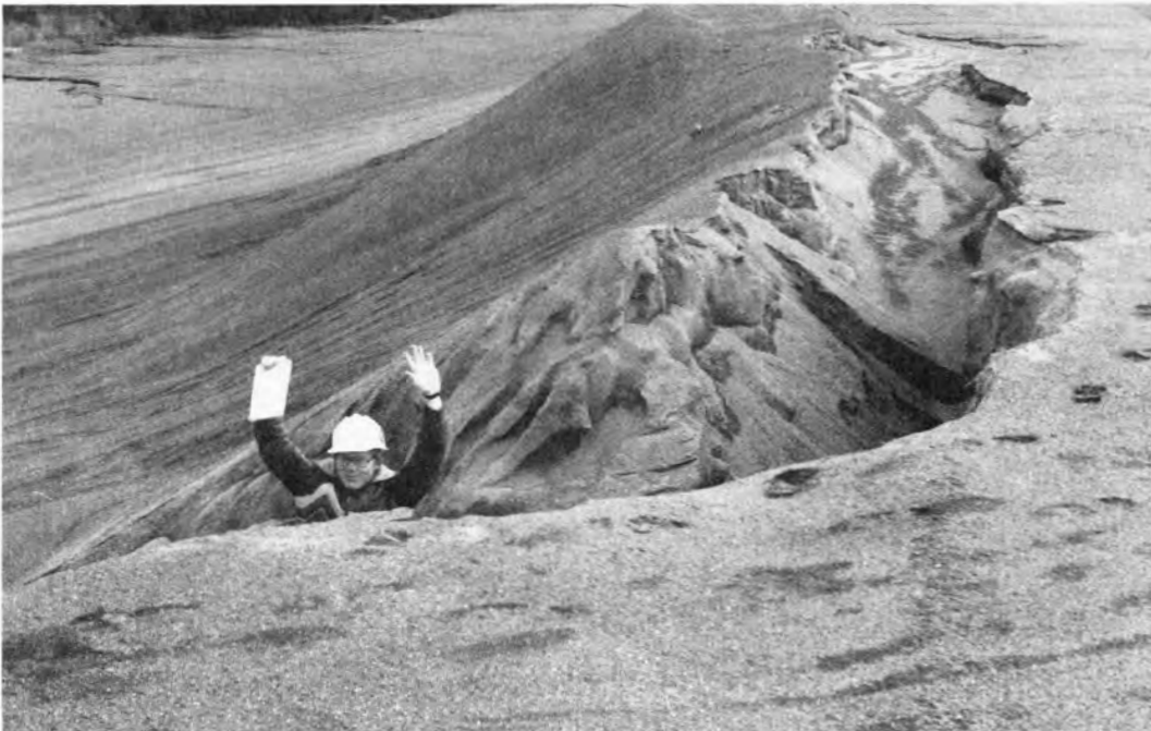
Figure 5-5. Routine dam inspection is a necessary part of a dam safety program. This rather dramatic erosion problem was identified during a routine inspection. Source: Minnesota Dept. of Natural Resources.
