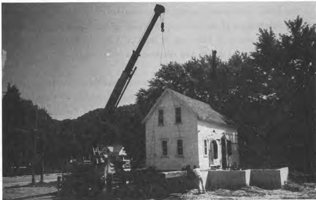
Figure 4-3. House behind levee in Soldier's Grove, Wisconsin being elevated after severe flooding in 1978. Source: T. Hirsch.
