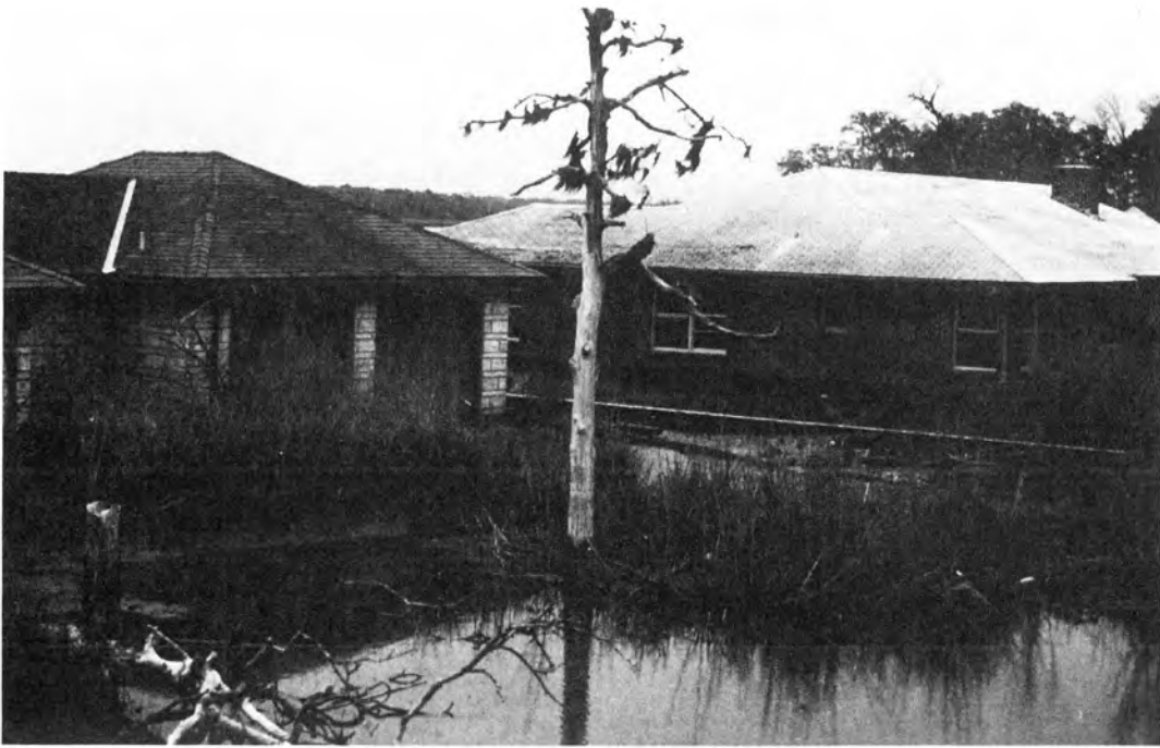
Figure 9-1. These houses in Brownwood Subdivision are flooded by daily tides because withdrawal of fluids has resulted in 2.5 meters of subsidence. Source: R. Platt.
